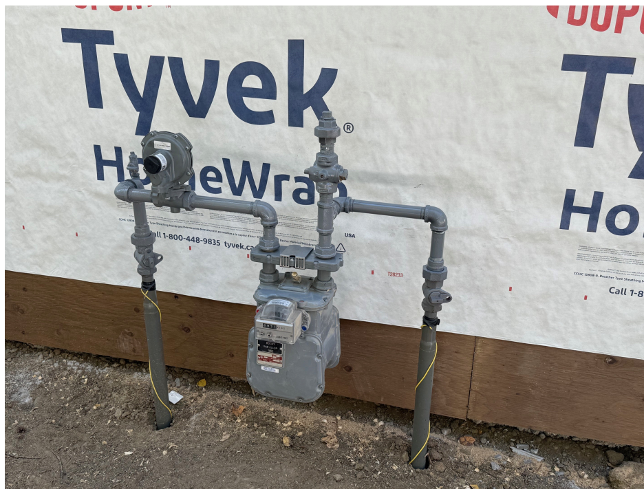
Typical low pressure .25 psi meter hang
