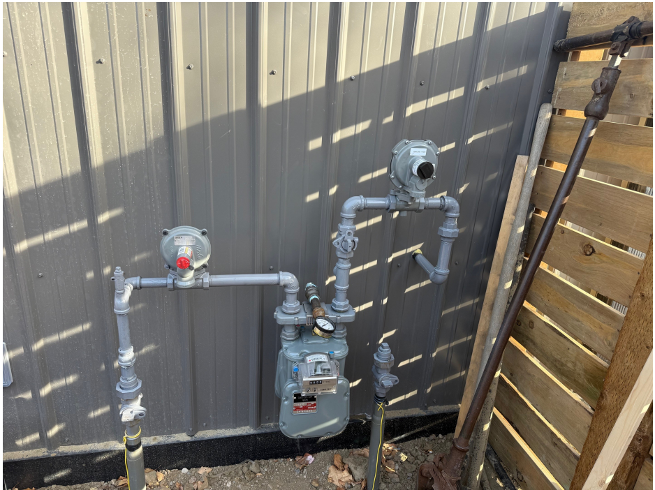
Typical high pressure 5 psi meter hang for additional buildings
