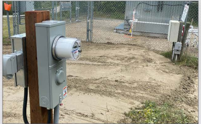
Uninterrupted power at an RMO
